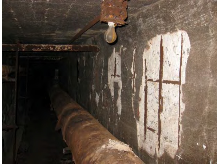
40. Tunnel's Damaged Walls (Concrete Spalled off & Rebars Corroded)
