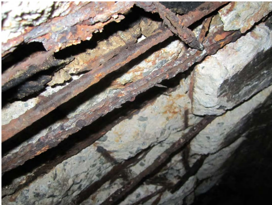
Picture #38- Deep spalling and extensive corrosion near Station 26
