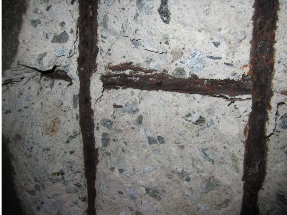
Picture #59- Spall with reinforcing steel with advanced corrosion occurring Section 20-21
