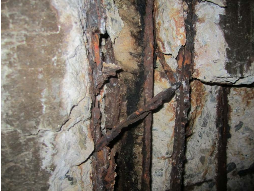
Picture #37- Delamination and severe reinforcing steel corrosion near Station 26
