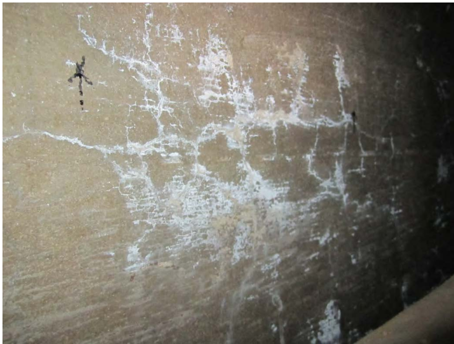
Picture #84- Many small cracks
