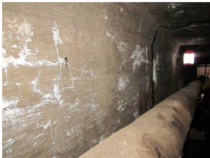
66. Tunnel Walls Delamination Concrete (Ready to Spall off)
