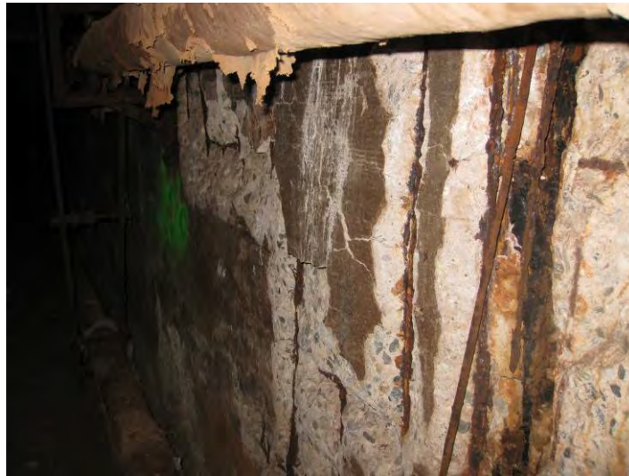
38. Tunnel's Damaged Walls (Concrete Spalled off & Rebars Corroded)
