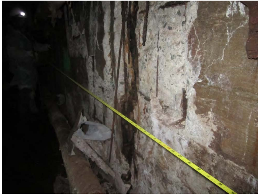
Picture #35- Spall in Section 25-26 with broken reinforcing steel and extensive section loss
