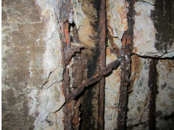
46. Tunnel's Damaged Walls (Concrete Spalled off & Rebars Corroded)
