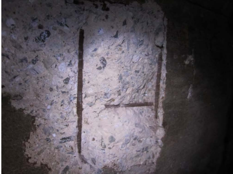
Picture #51- Spall near Station 19
