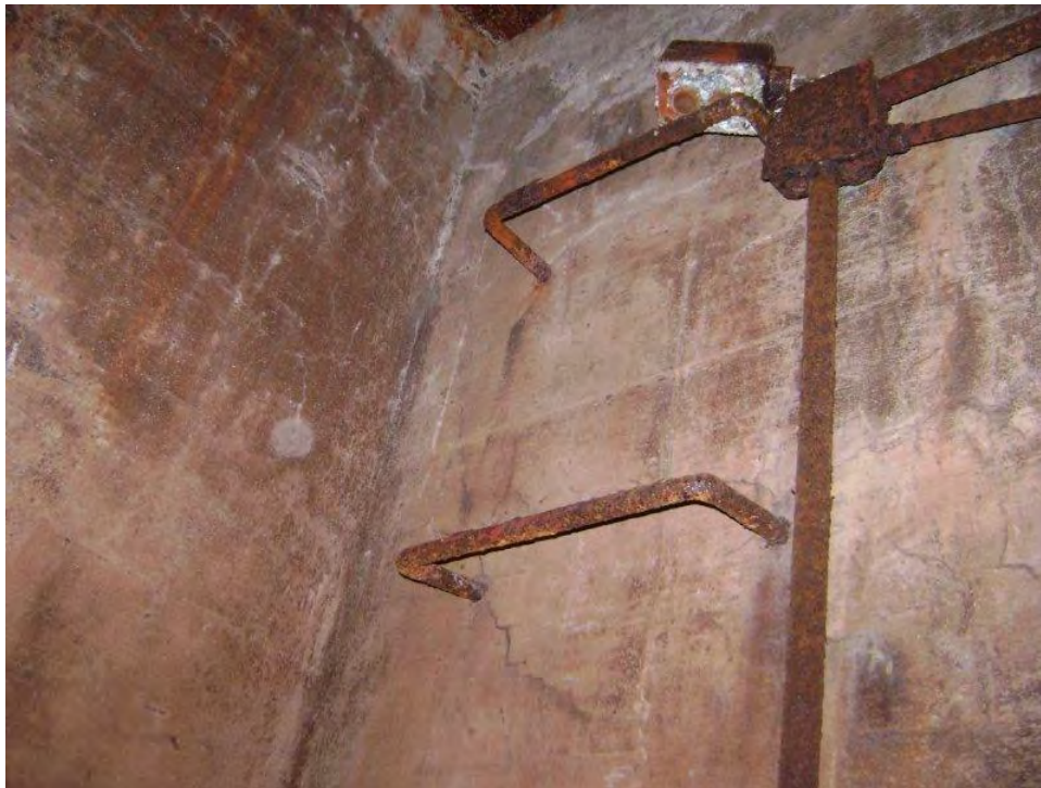
PHOTO 16: ELECTRICAL CONDUIT CORRODED
