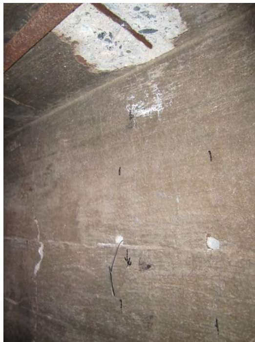
Picture #2- Ceiling spall
