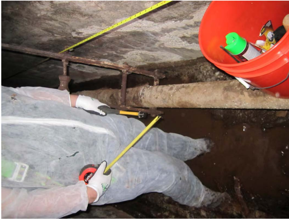
Picture #7- Water covered floor and soft concrete with shallow spalls Section 12-13
