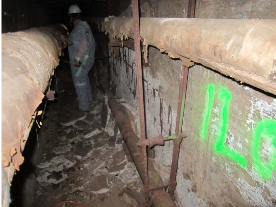
Picture #57- Severe spalling Section 20-21
