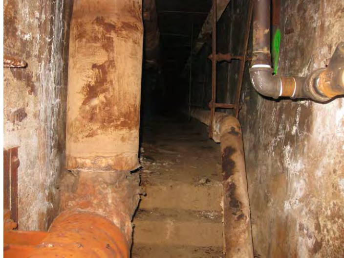
55. Tunnel Walls Delamination Concrete (Ready to Spall off)
