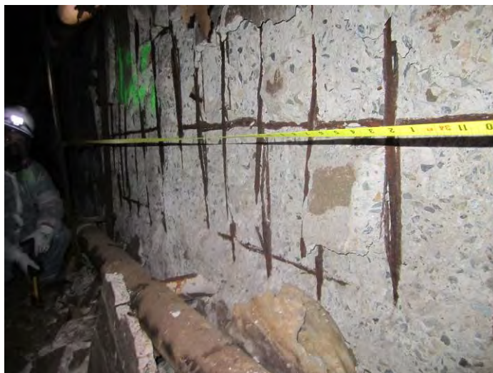
45. Tunnel's Damaged Walls (Concrete Spalled off & Rebars Corroded)
