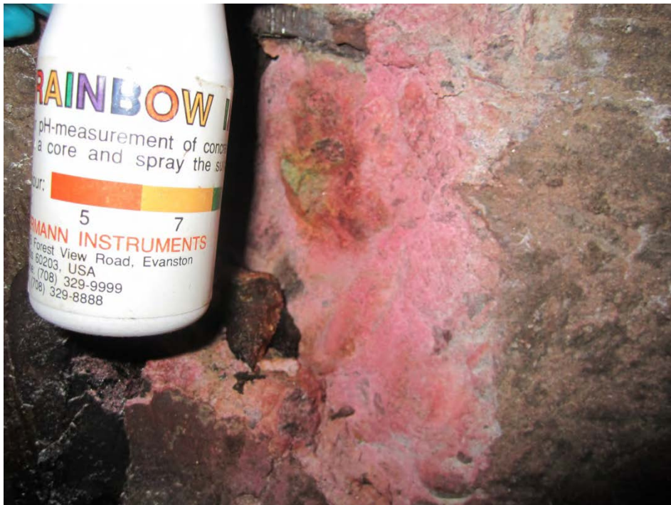
Picture #78- Spalled area indicating a PH of approximately 5
