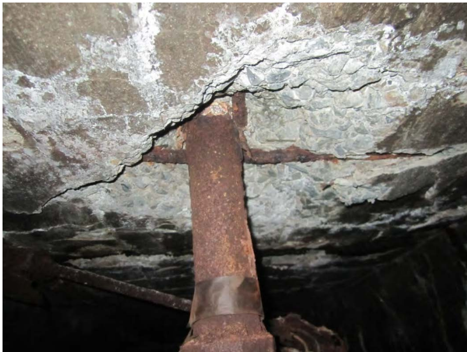
Picture #36- Ceiling delamination with corroded pipe, conduit, and reinforcing steel near Station 26
