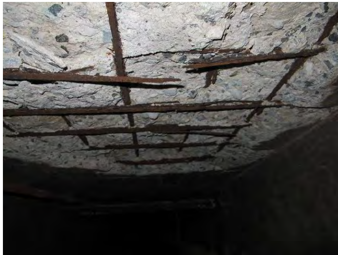
26. Tunnel's Damaged Ceiling (Concrete spalled off & rebars corroded)
