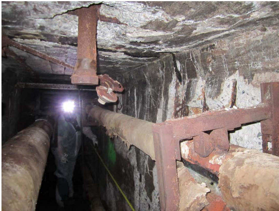
Picture #34- Damage tunnel section with spalling and heavy corrosion near Station 26
