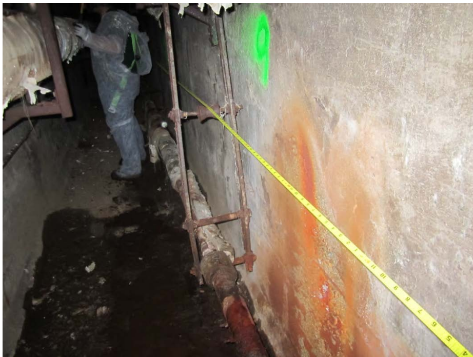
Picture #26- Damage from steam leak Section 8-9
