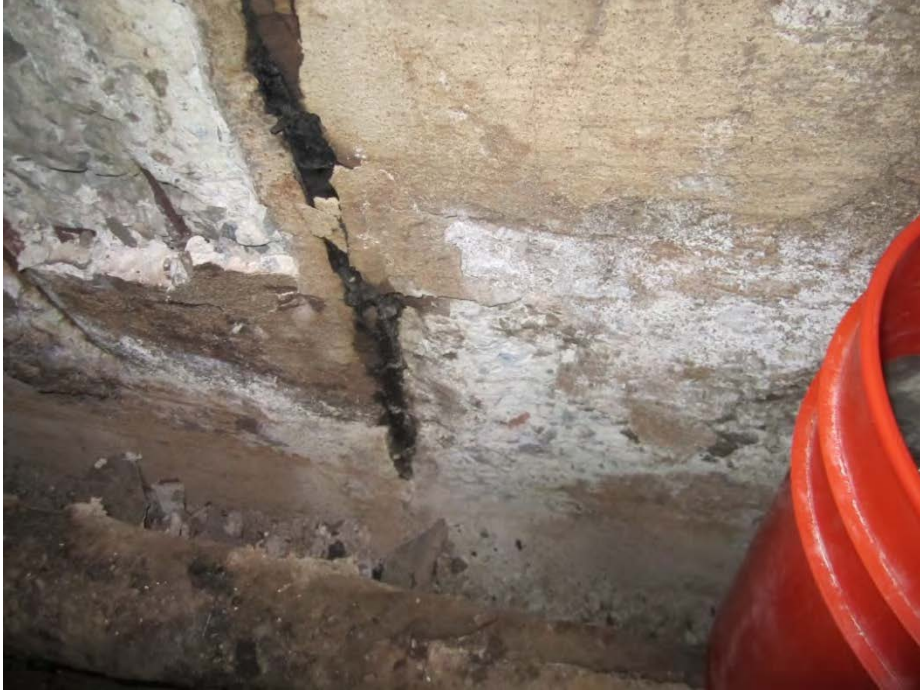
Picture #55- Spalling Section 19-20
