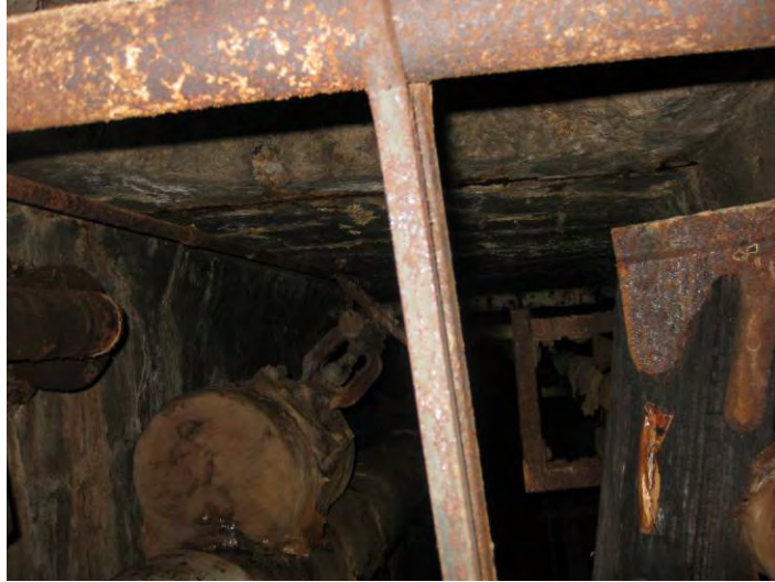
28. Tunnel's Damaged Ceiling & Shored
