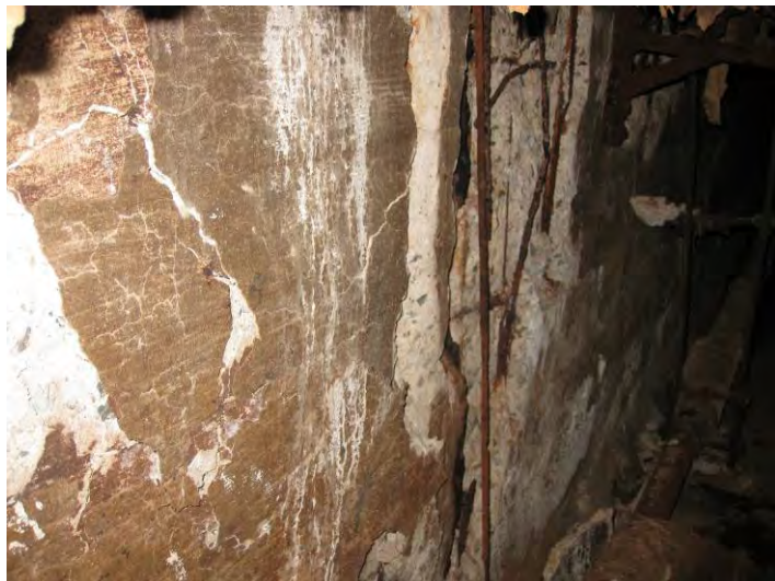
51. Tunnel Walls Delamination Concrete (Ready to Spall off)
