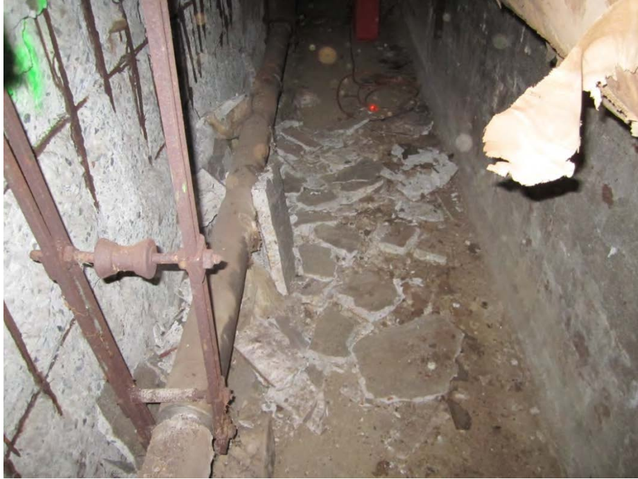
Picture #61- Spalling Section 20-21
