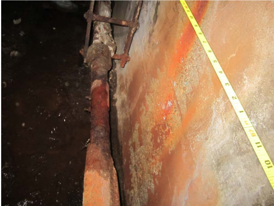
Picture #27- Damage from steam leak Section 8-9
