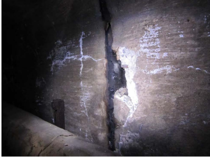
Picture #53- Spall next to leaking joint Section 19-20
