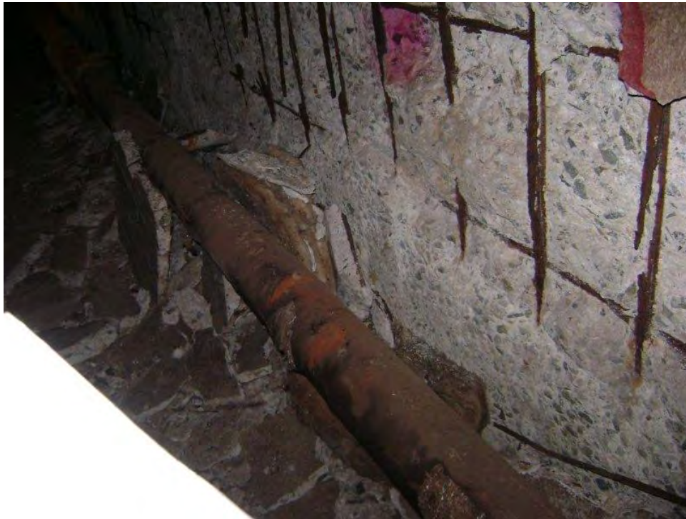
PHOTO 14: CONCRETE WALL FELL ON TOP OF STEAM CONDENSATE PIPE
