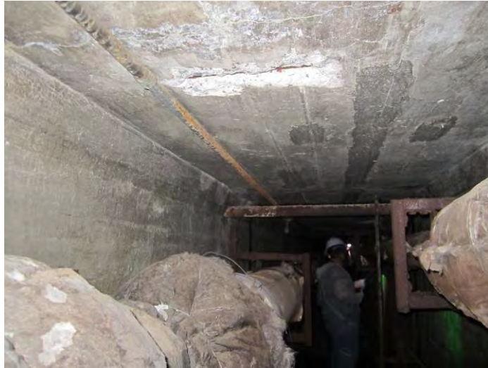
34. Tunnel's Ceiling Delamination (Concrete Ready to spall off)
