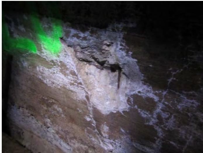
68. Tunnel Walls Delamination Concrete (Ready to Spall off)
