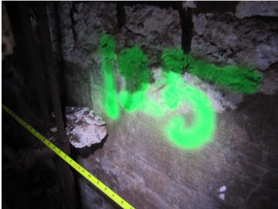
Picture #33- Spall with corroded reinforcing steel at Station 25
