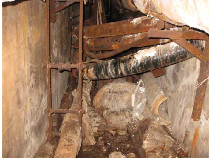
1. Tunnel Completely obstructed at Zonal Av.
