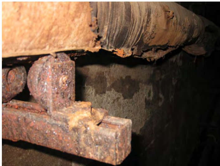
69. Tunnel Steam Pipe Support Completely Rusted & Not Adequately Anchored
