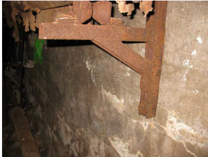
71. Tunnel Steam Pipe Support Completely Rusted & Not Adequately Anchored
