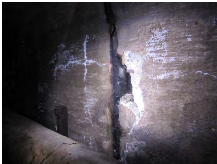
63. Tunnel Walls Delamination Concrete (Ready to Spall off)
