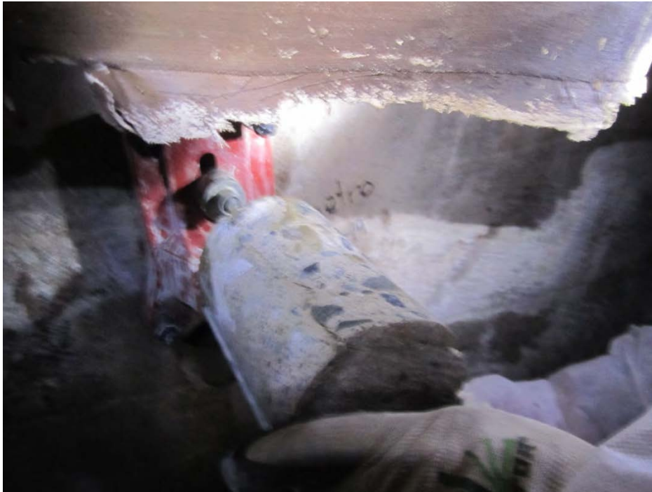
Picture #77- Petro13-14S visible crack
