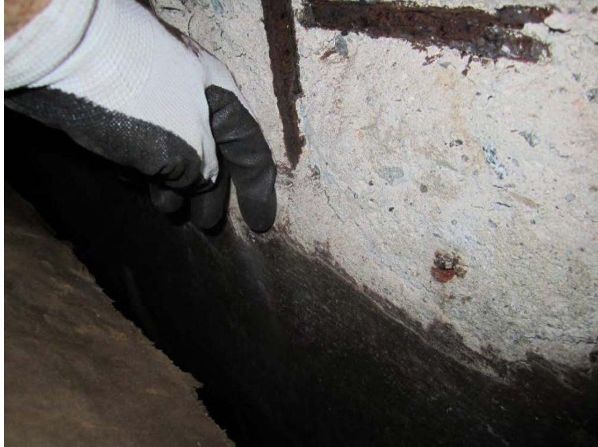
Picture #41- Spalling and soft concrete Section 35-36
