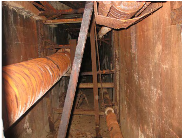
2. Tunnel Completely Obstructed at 100 FT Inside Juvenile Hall
