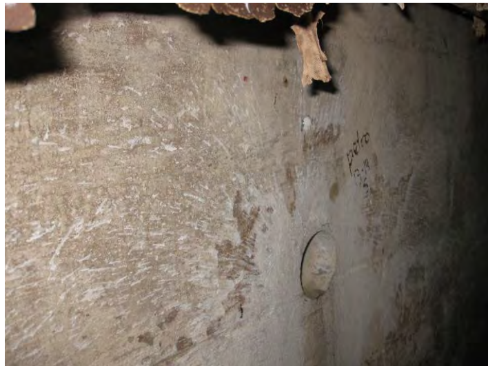
60. Tunnel Walls Delamination Concrete (Ready to Spall off)
