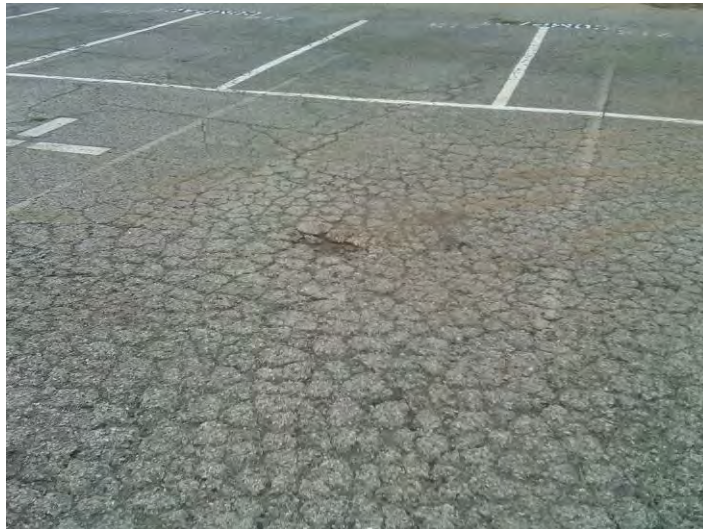
86. Damaged Surface parking Structure above the (E) Tunnel
