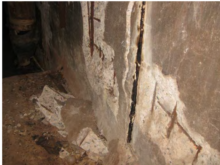
39. Tunnel's Damaged Walls (Concrete Spalled off & Rebars Corroded)
