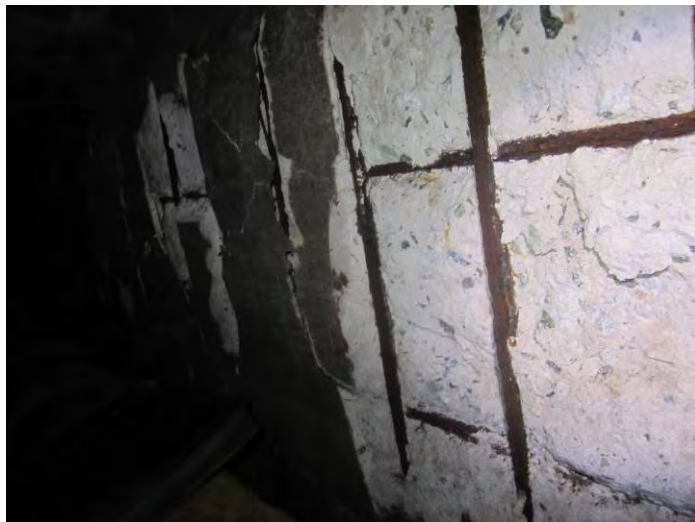
48. Tunnel's Damaged Walls (Concrete Spalled off & Rebars Corroded)
