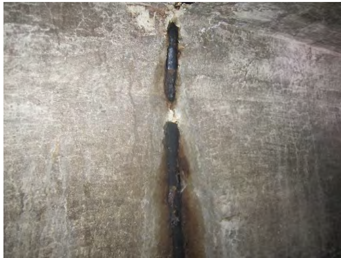
62. Tunnel Walls Delamination Concrete (Ready to Spall off)
