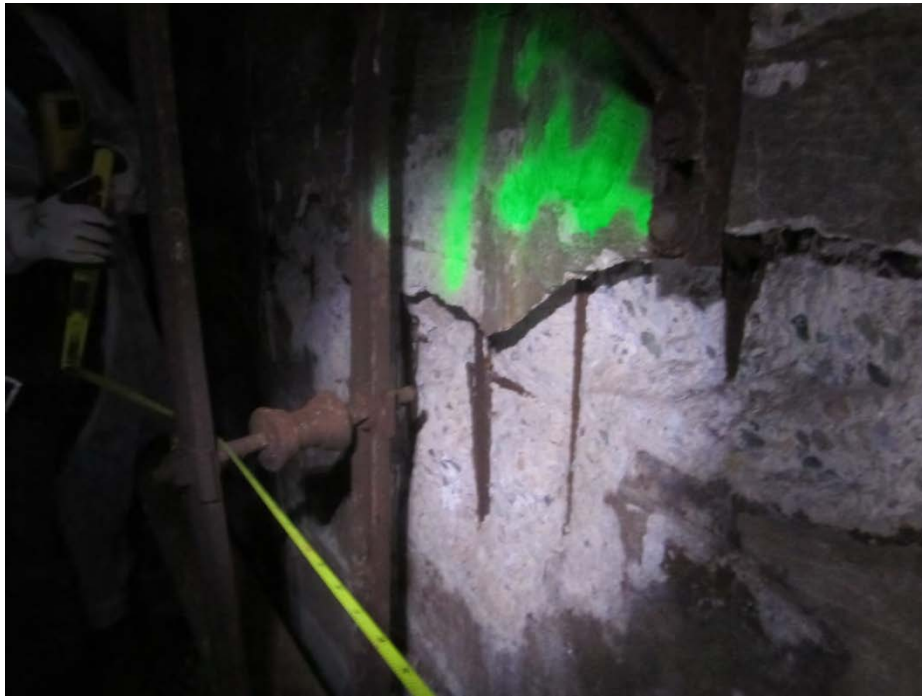
Picture #44- Spalling at Station 22
