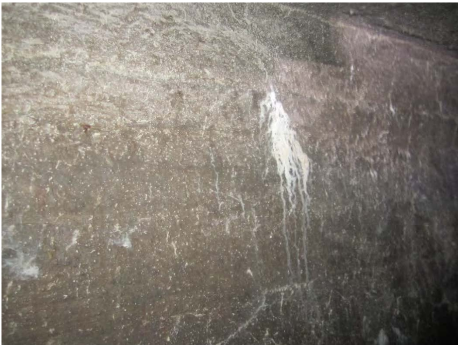
Picture #14- Efflorescent Section 3-4
