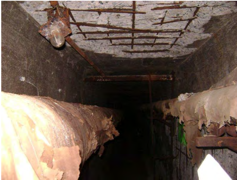
PHOTO 15: ELECTRICAL CONDUIT CORRODED
