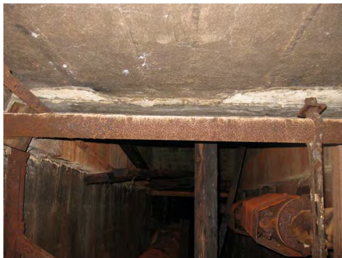
33. Tunnel's Ceiling Delamination (Concrete Ready to spall off)
