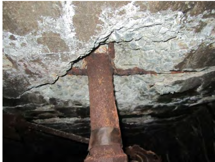
35. Tunnel's Ceiling Delamination (Concrete Ready to spall off)
