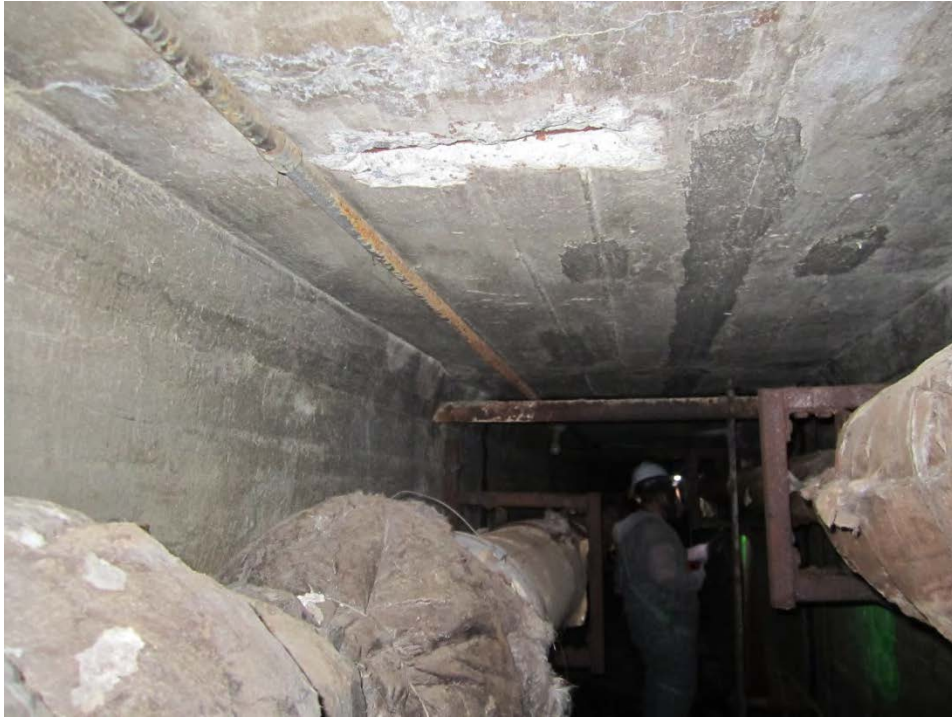
Picture #25- Ceiling spall Section 7-8
