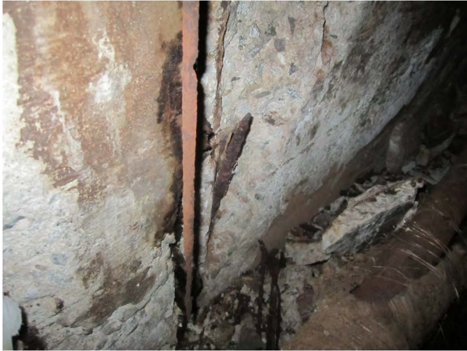
Picture #83- Spalling around a joint
