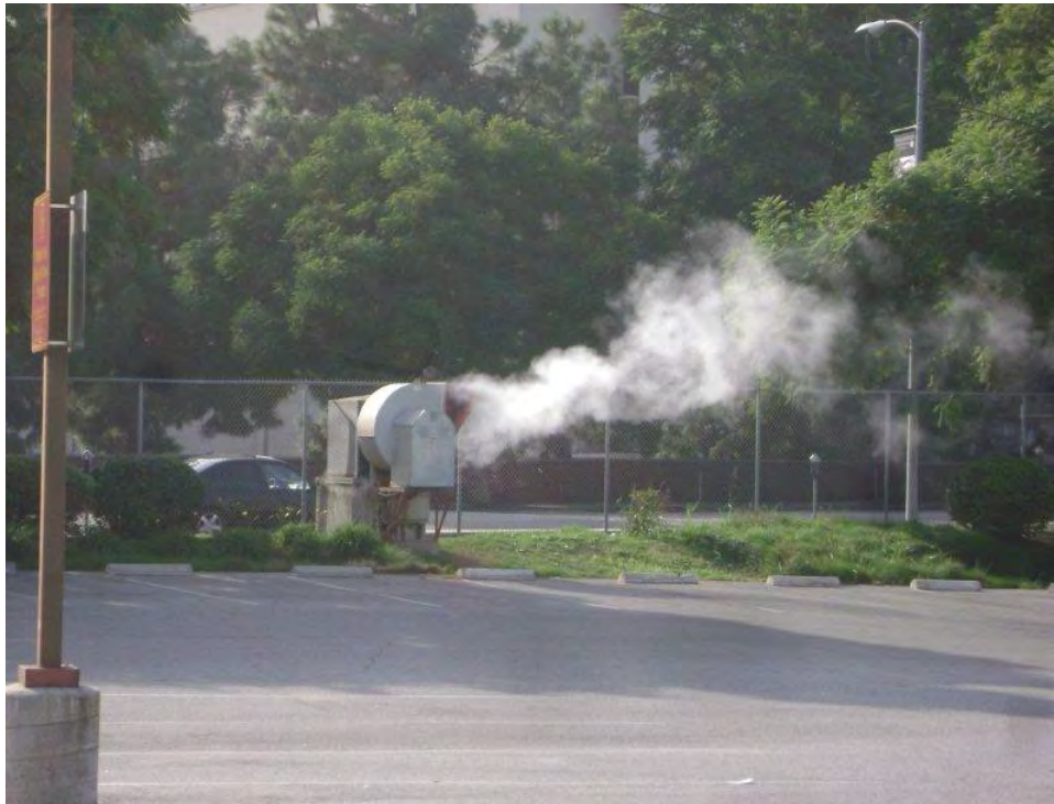
PHOTO 7: STEAM ESCAPING (EASILY OBSERVABLE) THRU EXHAUST FAN ON TOP OF MANHOLE AT ZONAL AVENUE
