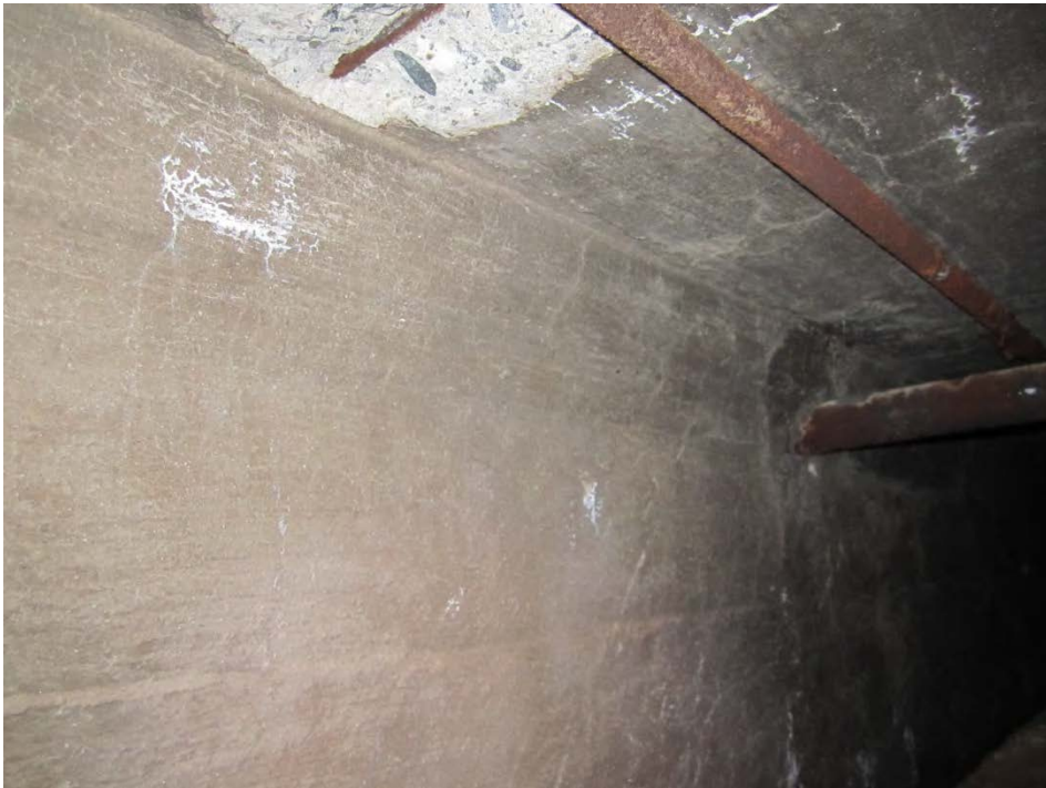
Picture #56- Ceiling spall Section 19-20
