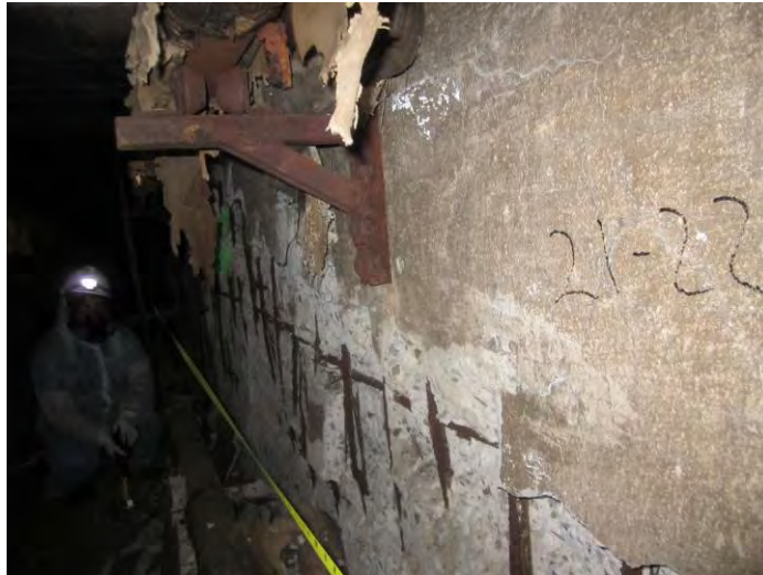
44. Tunnel's Damaged Walls (Concrete Spalled off & Rebars Corroded)
