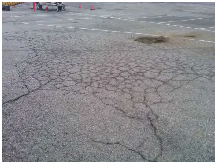
87. Damaged Surface parking Structure above the (E) Tunnel
