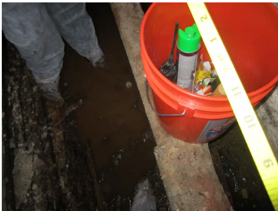
Picture #6- Water covering the tunnel floor in Section 12-13
