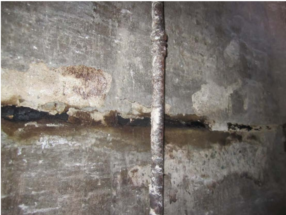
Picture #22- Deteriorated joint near Station 6
