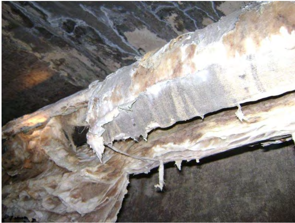
PHOTO 9: INSULATION IS FALLING APART
