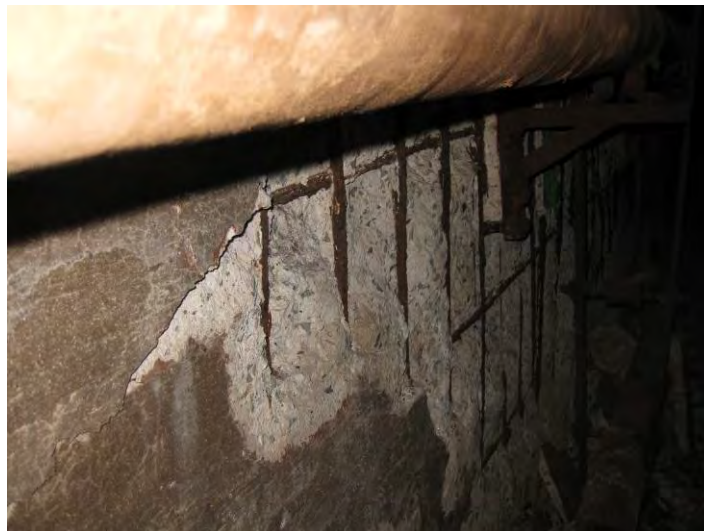
42. Tunnel's Damaged Walls (Concrete Spalled off & Rebars Corroded)
