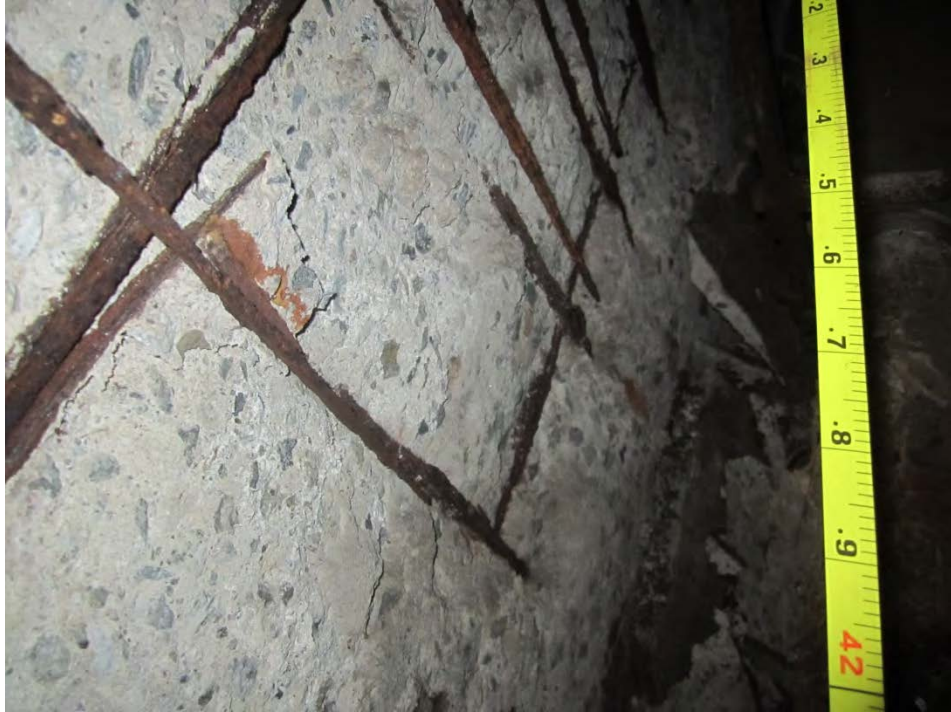
Picture #45- Spall with severe corrosion near station 22
