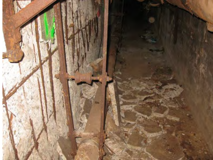
43. Tunnel's Damaged Walls (Concrete Spalled off & Rebars Corroded)
