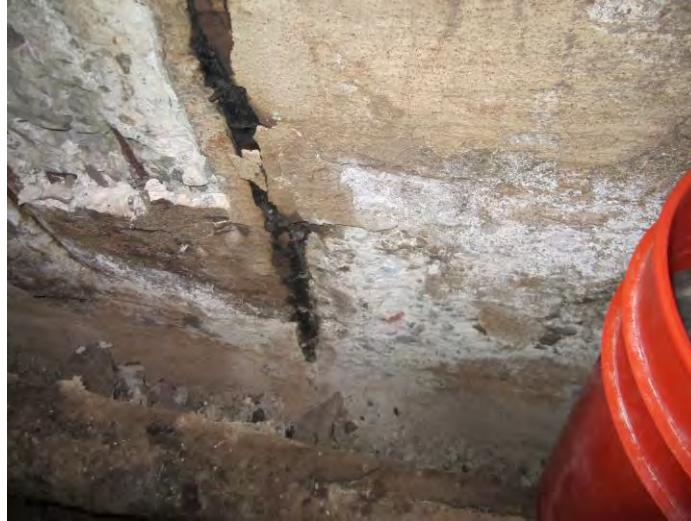
64. Tunnel Walls Delamination Concrete (Ready to Spall off)
