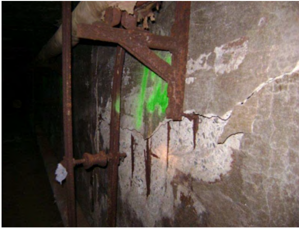
PHOTO 13: CONCRETE WALL SPALLED
