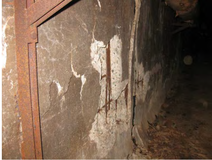
37. Tunnel's Damaged Walls (Concrete Spalled off & Rebars Corroded)
