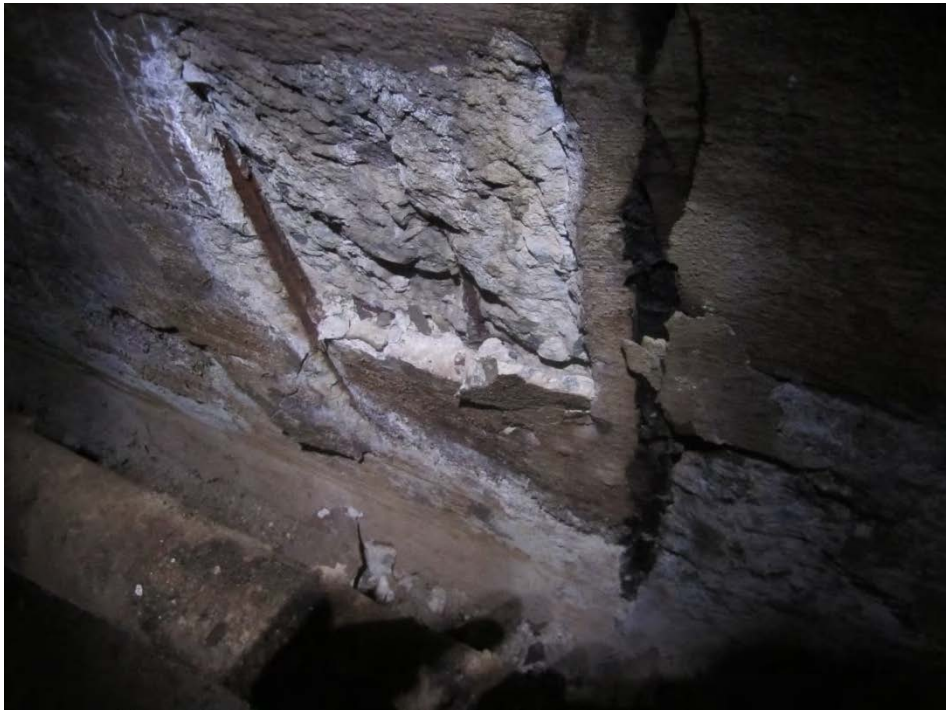
Picture #54- Spalling near joint Section 19-20
