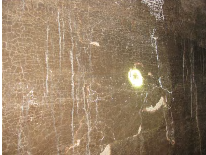
52. Tunnel Walls Delamination Concrete (Ready to Spall off)
