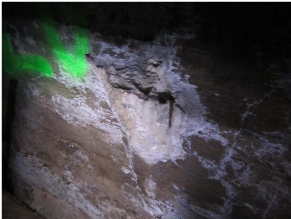
Picture #86- Spall around Station 20
