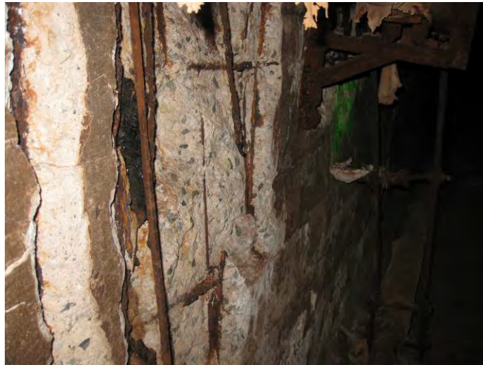
41. Tunnel's Damaged Walls (Concrete Spalled off & Rebars Corroded)
