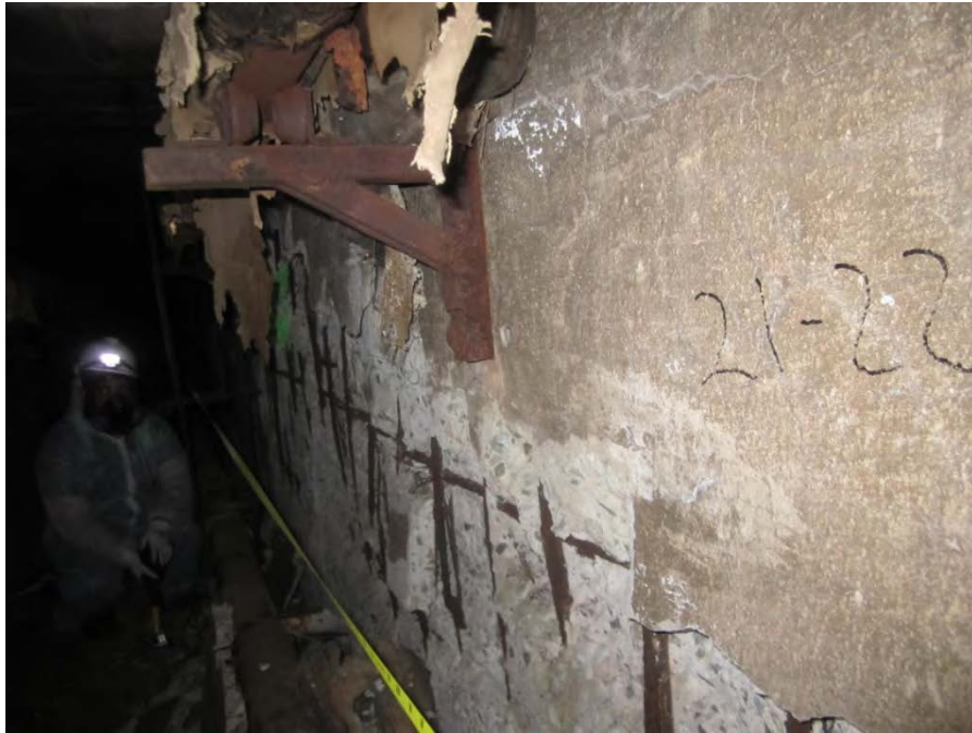
Picture #31- Spall with exposed corroded reinforcing steel Section 21-22
