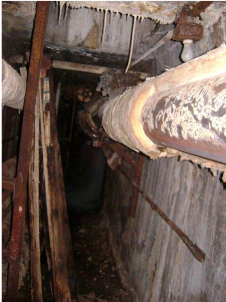
PHOTO 4: STEAM PIPE LEAKAGE NEAR MANHOLE AT ZONAL AVENUE
