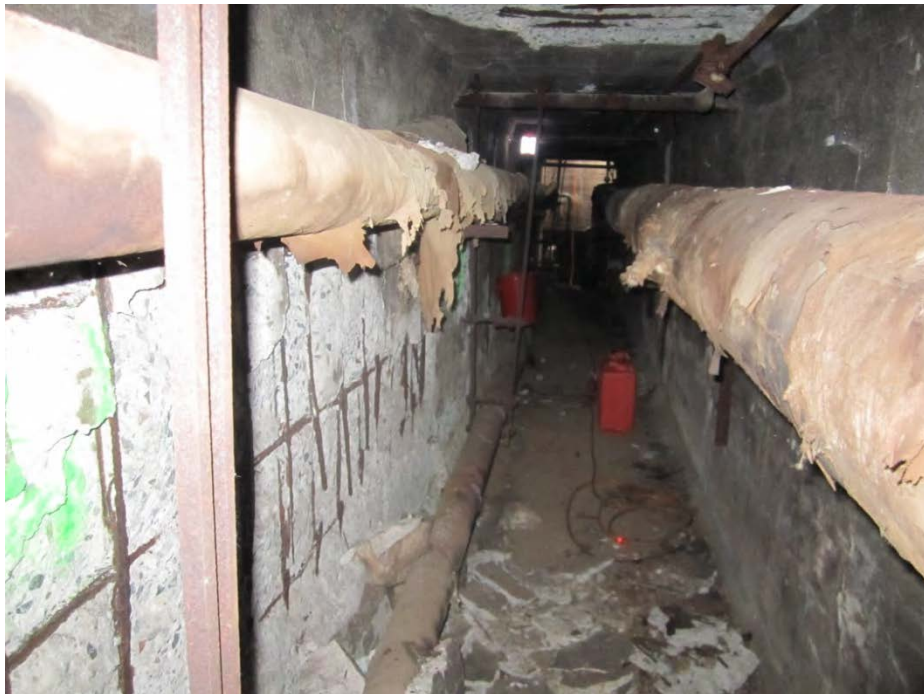
Picture #60- Spalling Section 20-21
