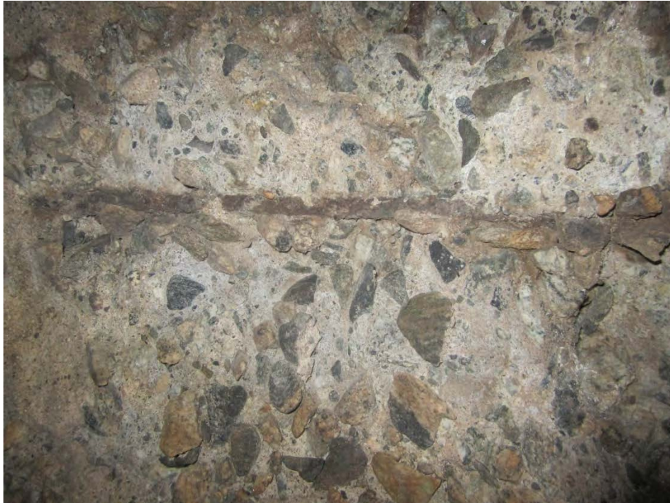
Picture #29- Exposed reinforcing steel Section 15-16
