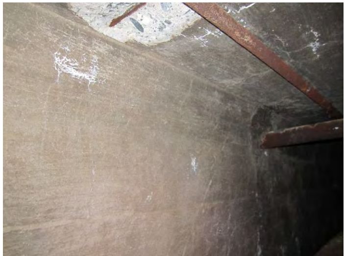
30. Tunnel's Damaged Ceiling (Concrete spalled off & rebars corroded)
