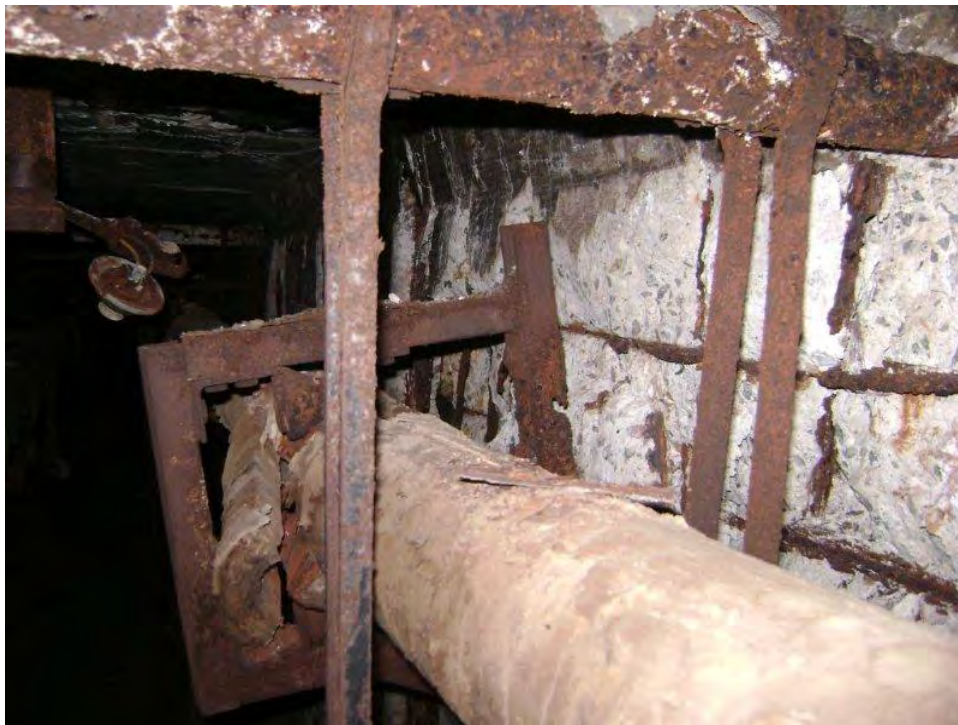
PHOTO 12: STEAM SUPPORT NOT PROPERLY ANCHORED OR SECURED TO CONCRETE WALL
