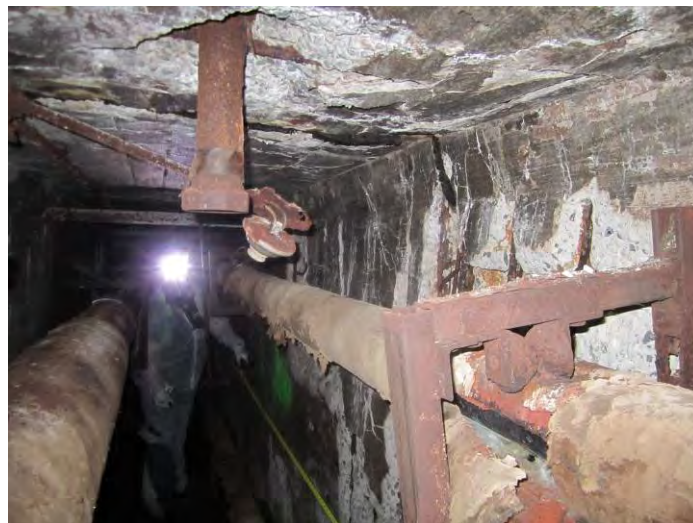
75. Tunnel Steam Pipe Support Completely Rusted & Not Adequately Anchored
