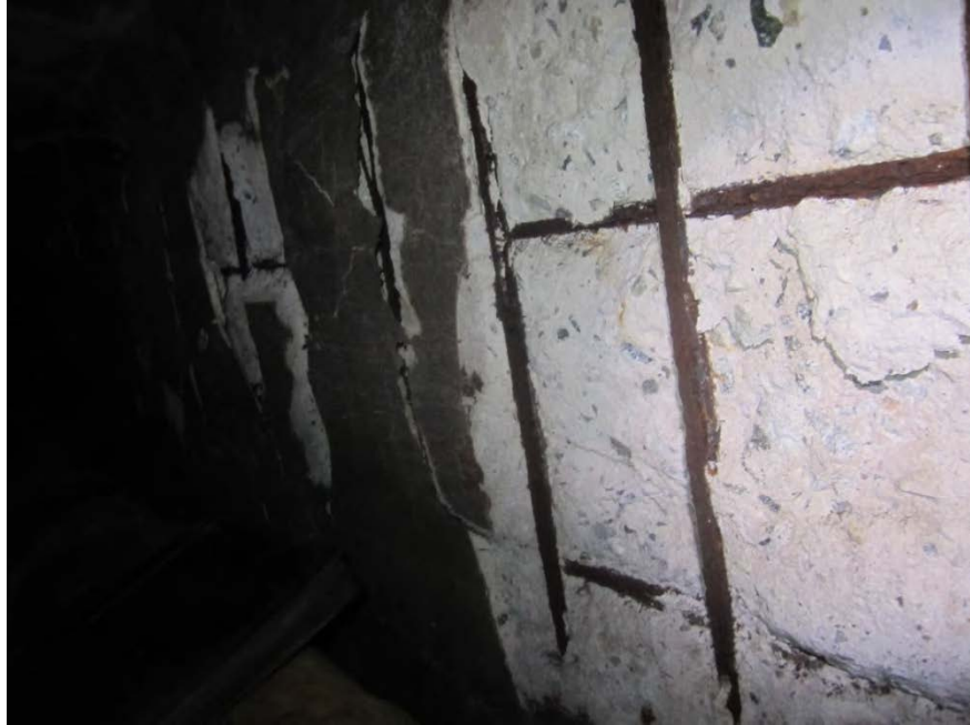
Picture #39- Delamination and spalling Section 35-36
