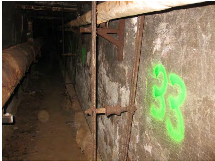
59. Tunnel Walls Delamination Concrete (Ready to Spall off)
