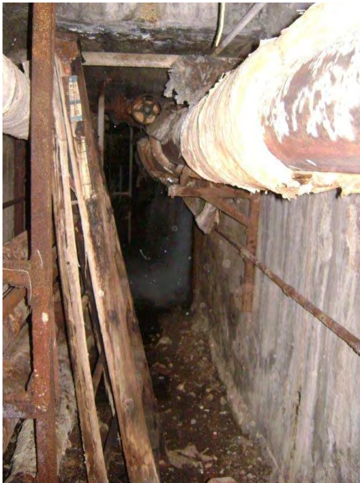
PHOTO 5: TEAM PIPE LEAKAGE NEAR MANHOLE AT ZONAL AVENUE
