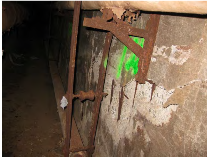
70. Tunnel Steam Pipe Support Completely Rusted & Not Adequately Anchored
