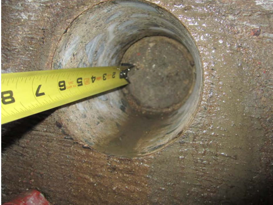
Picture #63- Core Hole from compressive strength core S19-20 on north wall approximately 5-3/8" thick
