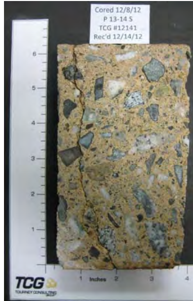
Figure 7 – Core P13-14S after staining with phenolphthalein showing lack of pink staining through the entire section of the core
