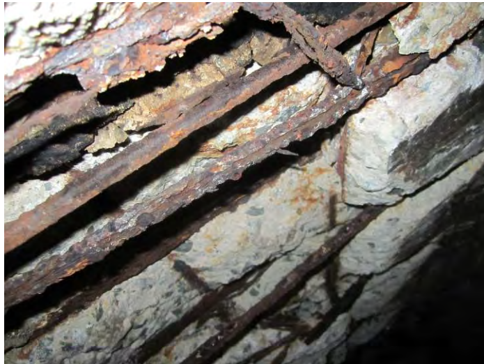
47. Tunnel's Damaged Walls (Concrete Spalled off & Rebars Corroded)
