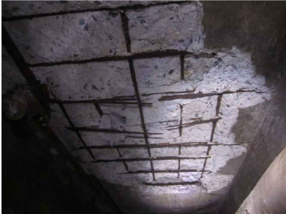
Picture #91- Ceiling spall near Station 20
