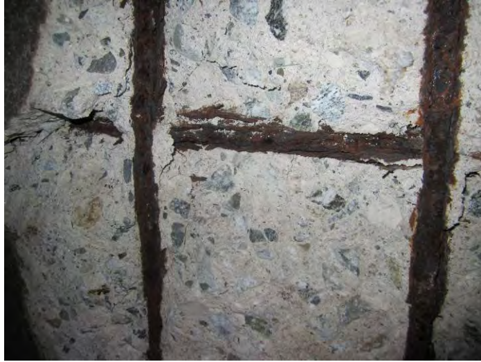
49. Tunnel's Damaged Walls (Concrete Spalled off & Rebars Corroded)
