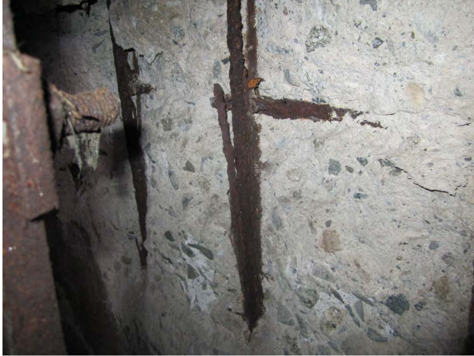
Picture #43- Spalling and corroded rebar Section 22-23
