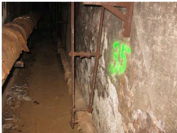
57. Tunnel Walls Delamination Concrete (Ready to Spall off)
