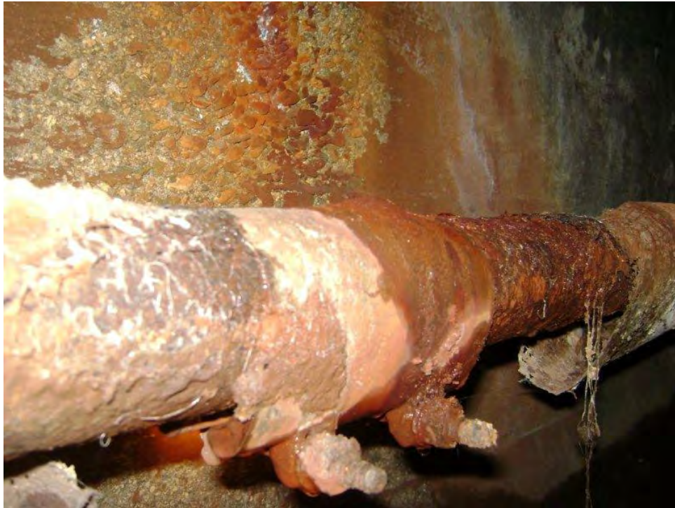
PHOTO 2: STEAM CONDENSATE PIPE LEAKAGE
