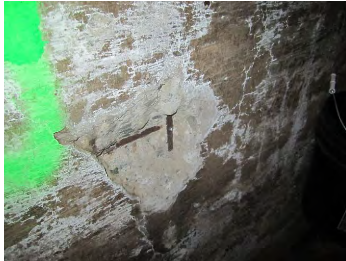
65. Tunnel Walls Delamination Concrete (Ready to Spall off)
