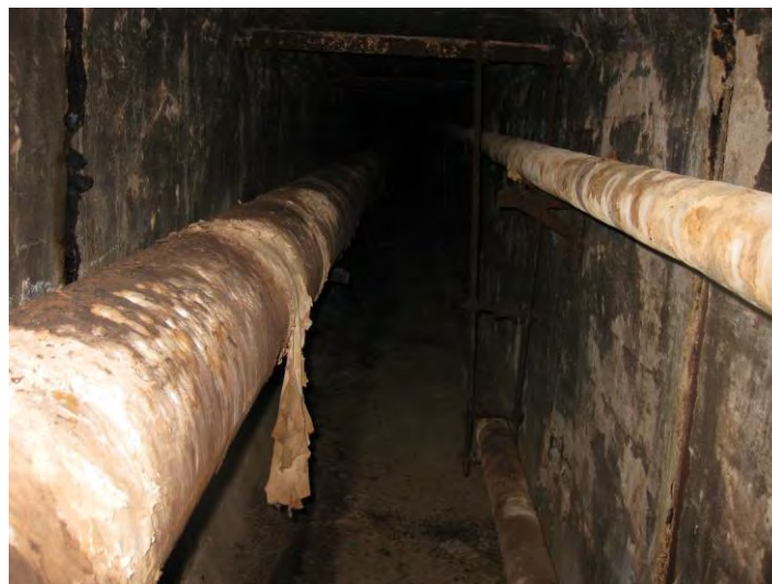
54. Tunnel Walls Delamination Concrete (Ready to Spall off)
