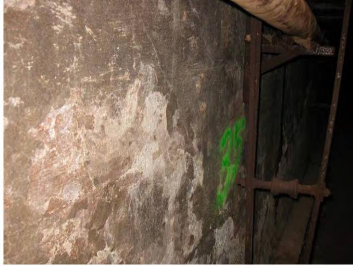
58. Tunnel Walls Delamination Concrete (Ready to Spall off)
