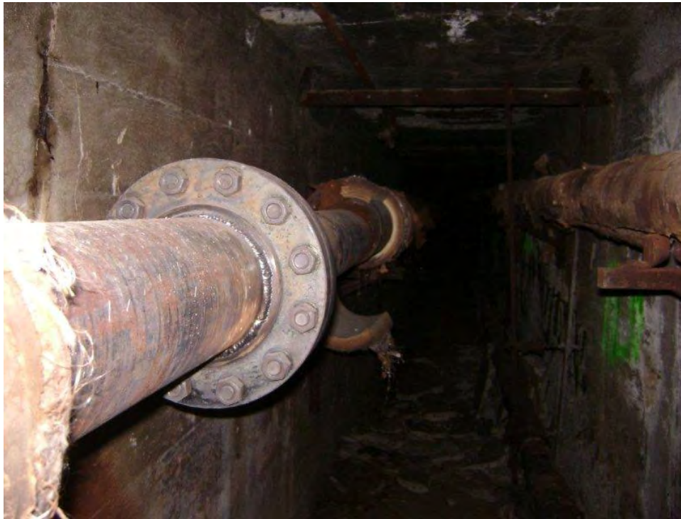
PHOTO 11: INSULATION MISSING FOR STEAM SUPPLY PIPE
