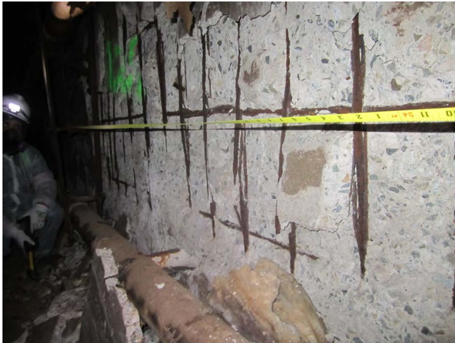
Picture #32- Spall with exposed corroded reinforcing steel Section 21-22
