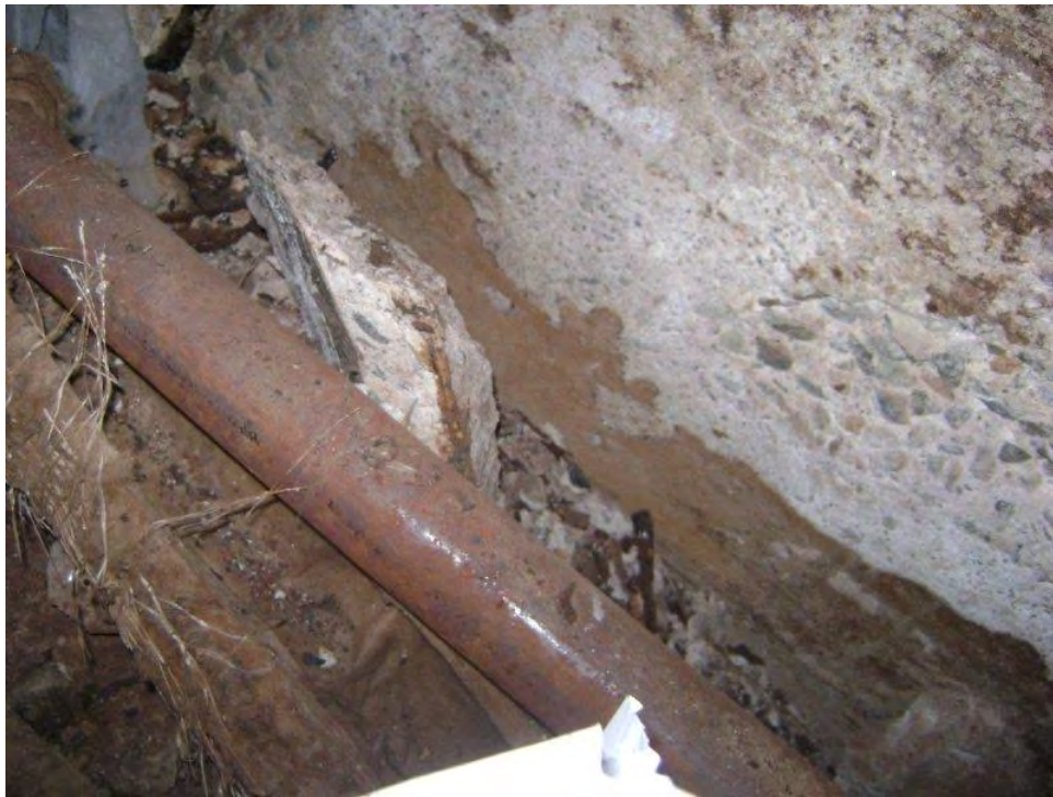
PHOTO 10: INSULATION IS FALLING APART
