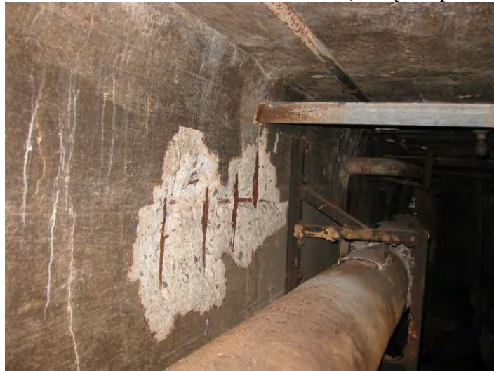
56. Tunnel Walls Delamination Concrete (Ready to Spall off)
