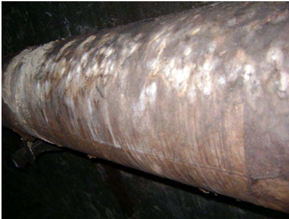
PHOTO 8: STEAM PIPE INSULATED WITH ASBESTOS
