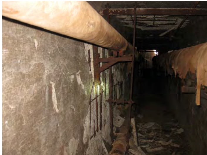
53. Tunnel Walls Delamination Concrete (Ready to Spall off)
