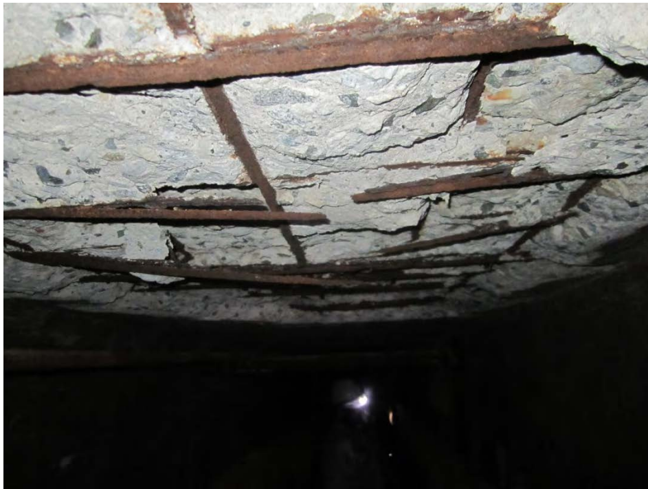
Picture #58- Ceiling spall with broken corroded reinforcement steel Section 20-21
