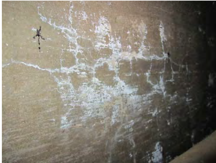
67. Tunnel Walls Delamination Concrete (Ready to Spall off)
