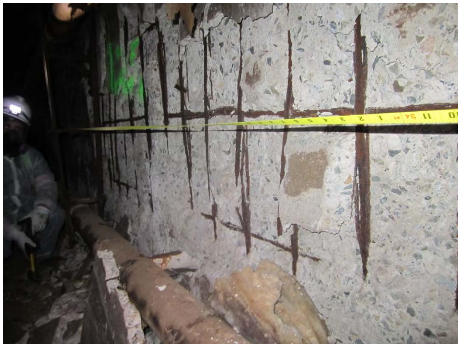
Figure 1 - Severely corroded reinforcing in spall at Station 21-22
