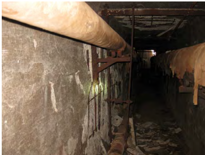
29. Tunnel's Damaged Ceiling (Concrete spalled off & rebars corroded)
