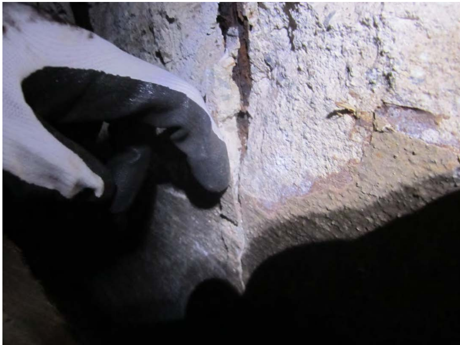
Picture #40- Spalling and soft concrete Section 35-36
