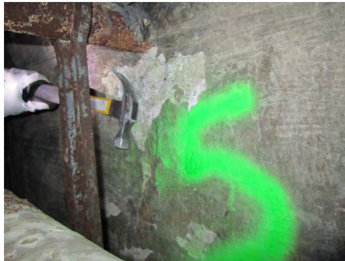
74. Tunnel Steam Pipe Support Completely Rusted & Not Adequately Anchored
