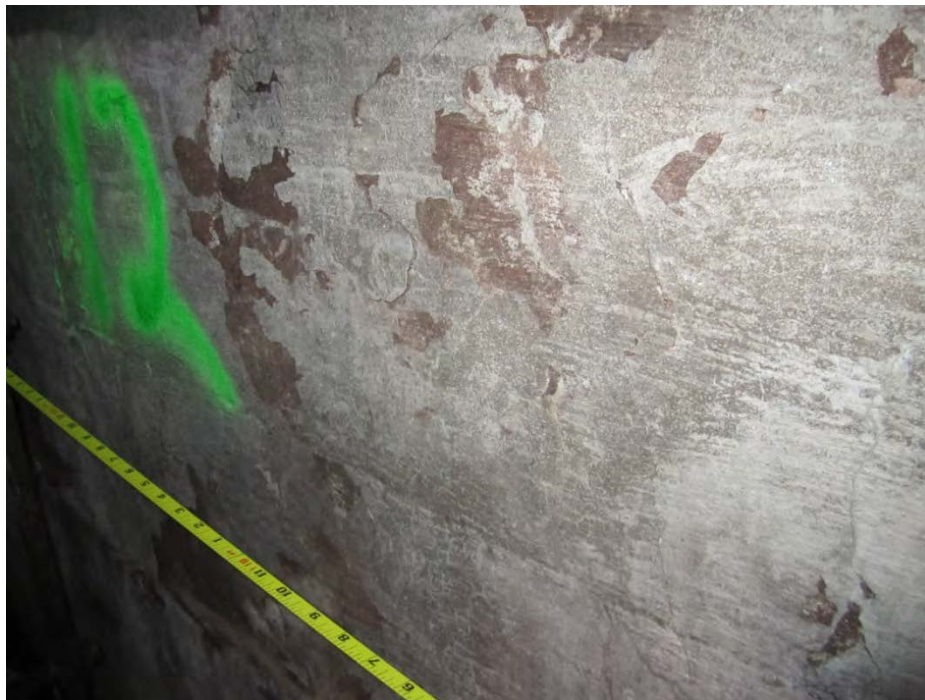
Picture #4- Soft concrete with small cracks in Section 11-12
