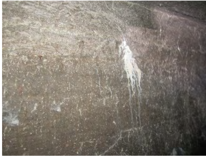
61. Tunnel Walls Delamination Concrete (Ready to Spall off)
