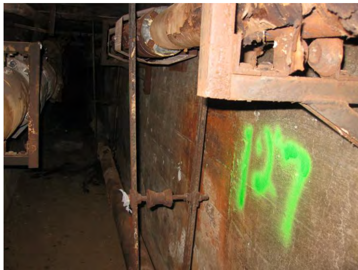
72. Tunnel Steam Pipe Support Completely Rusted & Not Adequately Anchored 4
