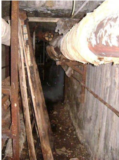
73. Tunnel Steam Pipe Support Completely Rusted & Not Adequately Anchored
