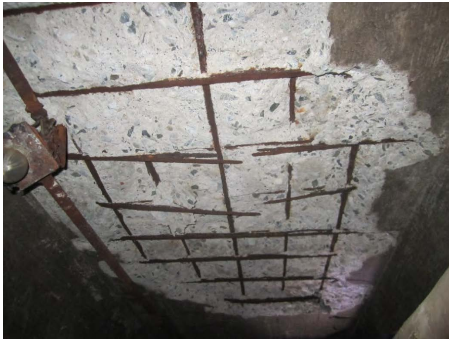
Picture #92- Ceiling Spall near Station 20
