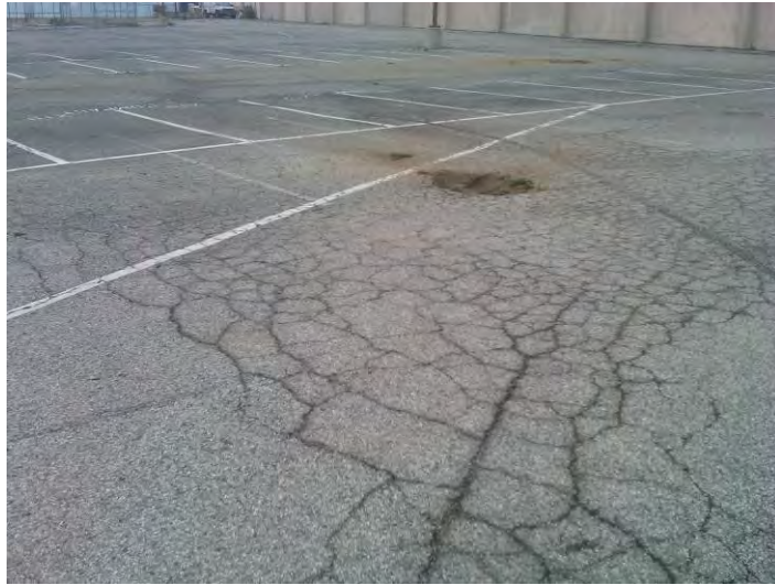
85. Damaged Surface parking Structure above the (E) Tunnel
