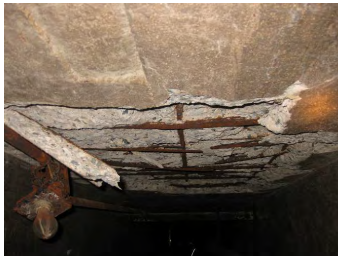
27. Tunnel's Damaged Ceiling (Concrete spalled off & rebars corroded)
