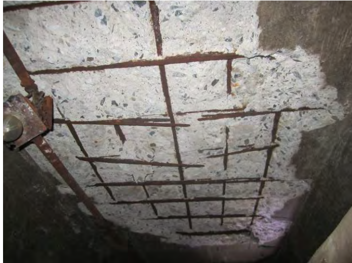
31. Tunnel's Damaged Ceiling (Concrete spalled off & rebars corroded)
