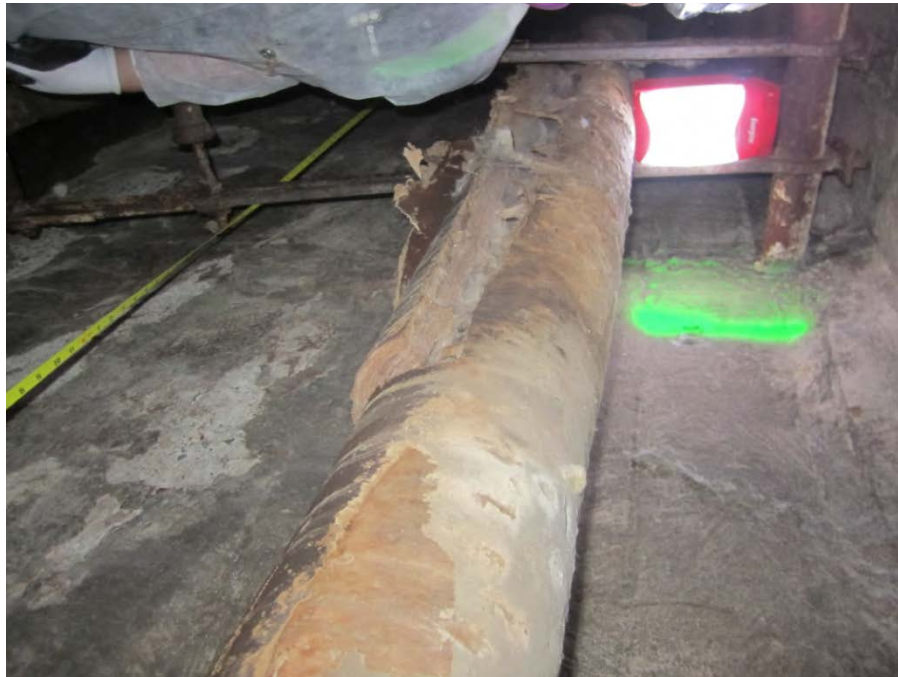
Picture #5- Soft concrete and shallow spalls in Section 0-1
