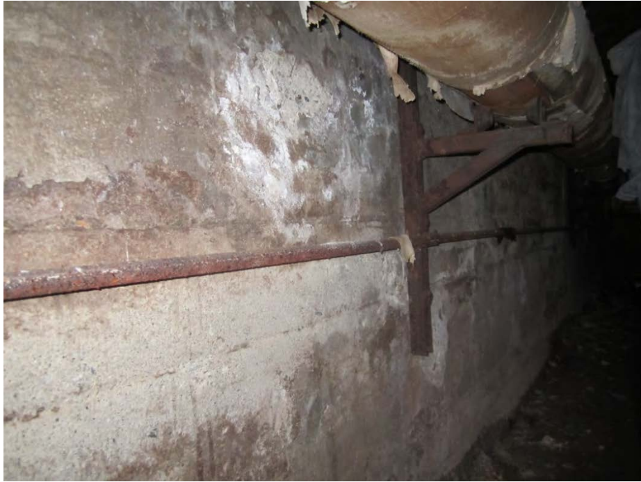
Picture #85- Soft flakey concrete
