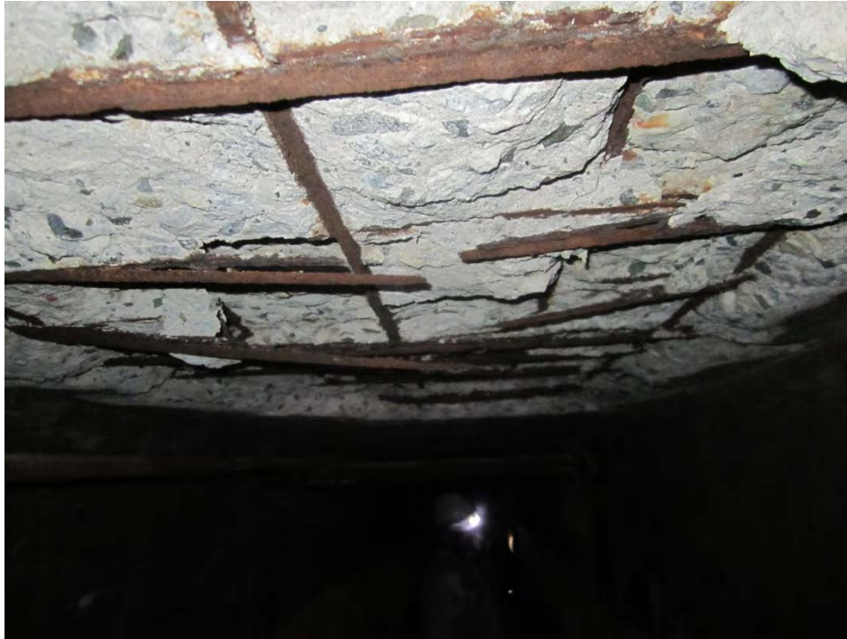
Figure 2 - Severely corroded tunnel ceiling slab reinforcement
