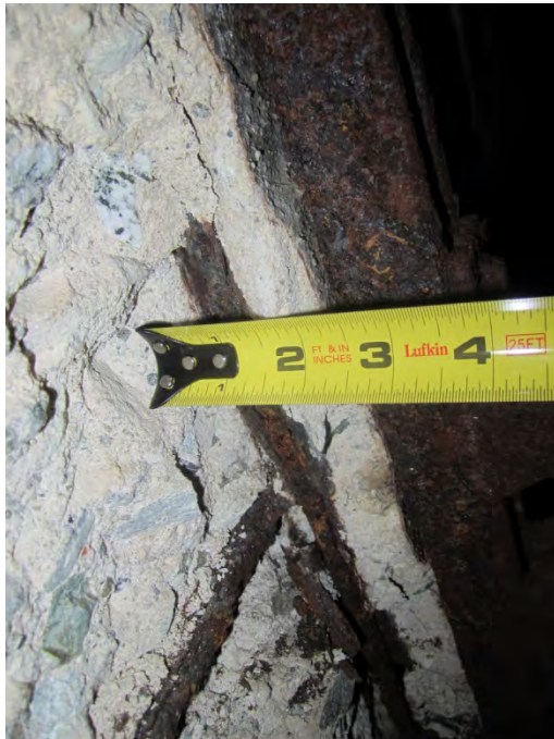
Picture #1-Approximate 2.5" thick spall
