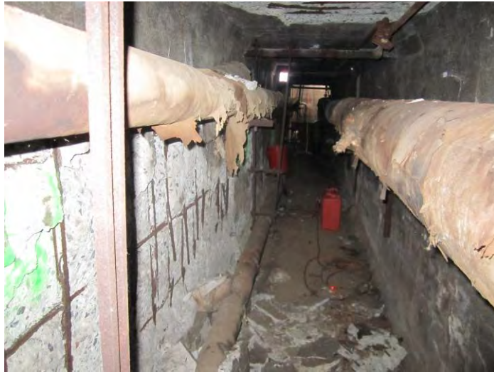
50. Tunnel's Damaged Walls (Concrete Spalled off & Rebars Corroded)
