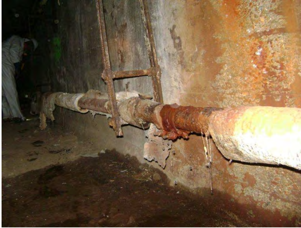
PHOTO 1: STEAM CONDENSATE PIPE LEAKAGE
