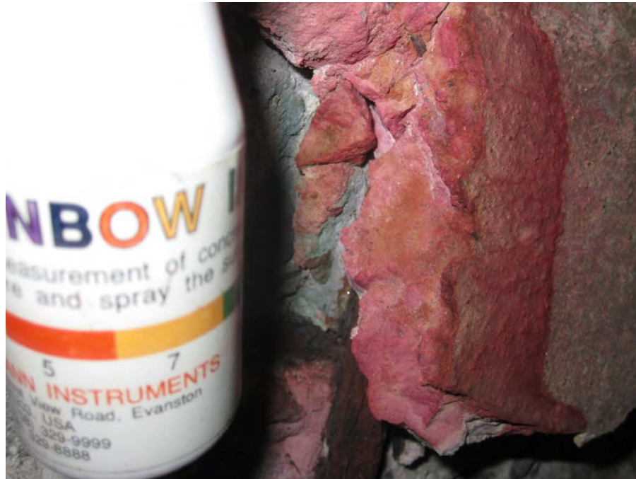
Picture #3- Spall sprayed with rainbow indicator around a 6 pH
