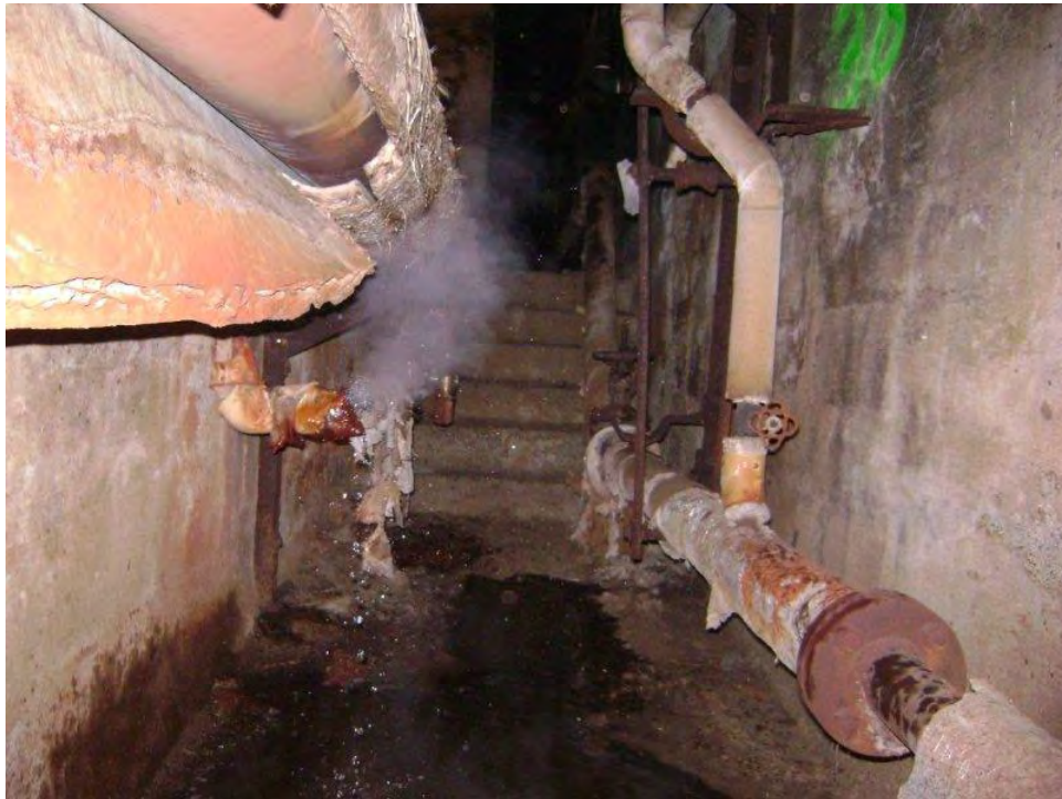
PHOTO 3: STEAM CONDENSATE PIPE LEAKAGE AS IT HEADS TO JUVENILE HALL
