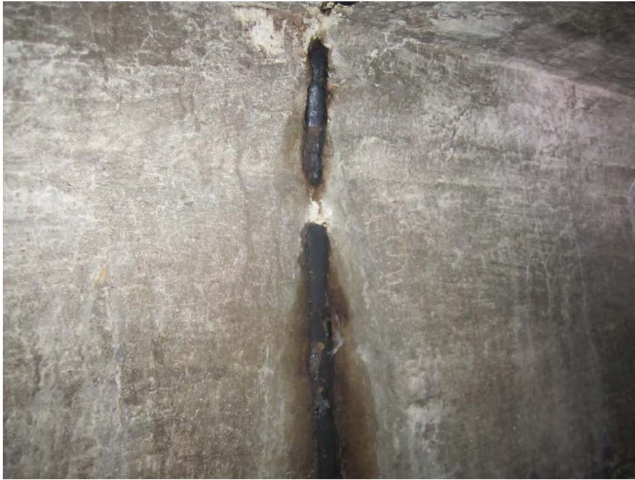
Picture #23- Deteriorated joint near Station 6
