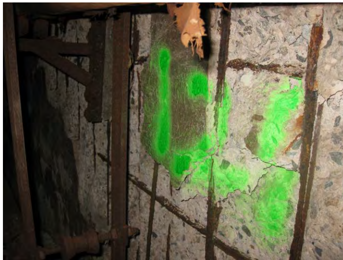
36. Tunnel's Damaged Walls (Concrete Spalled off & Rebars Corroded)
