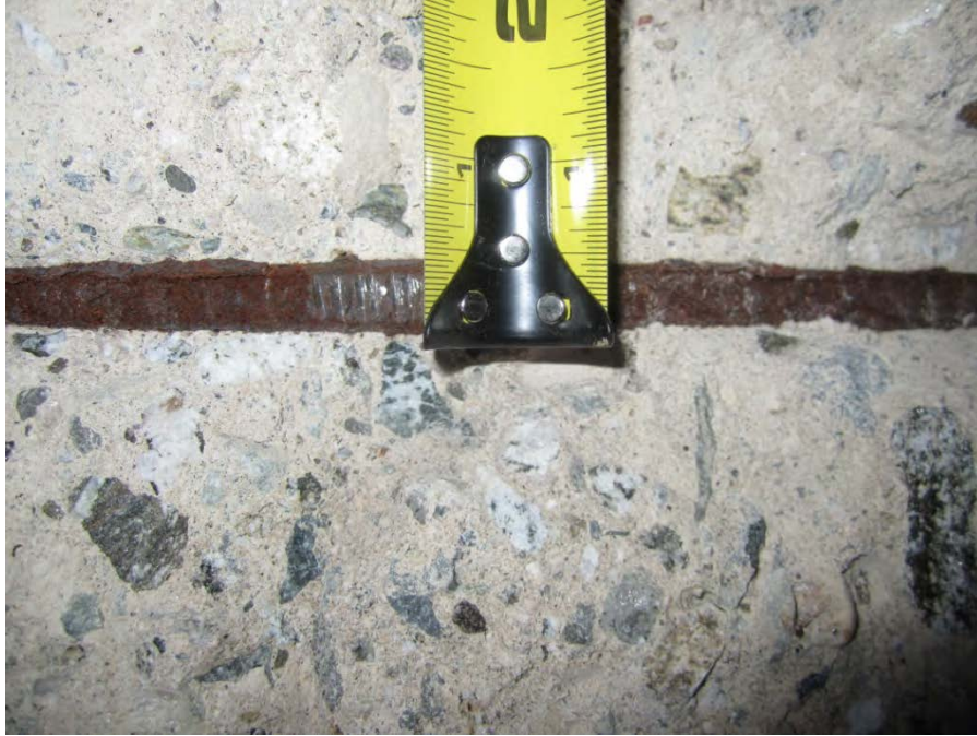
Picture #49- Exposed square Reinforcing bar 3/8"
