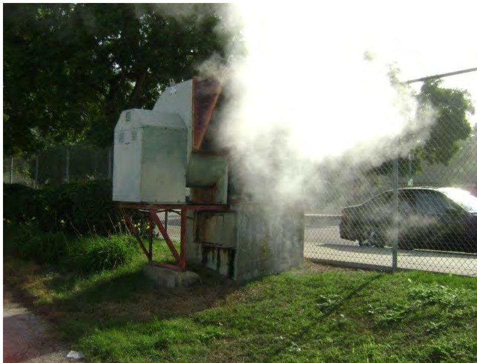
PHOTO 6: STEAM ESCAPING (EASILY OBSERVABLE) THRU EXHAUST FAN ON TOP OF MANHOLE AT ZONAL AVENUE
