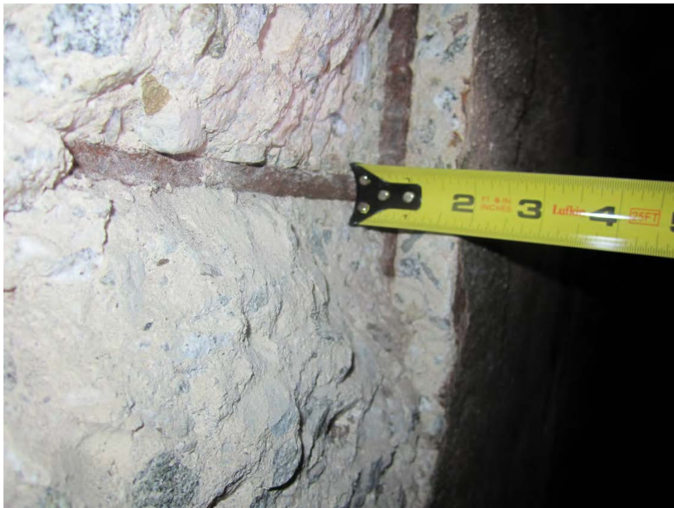
Picture #52- Spall depth approximately 1-3/4" near Station 19
