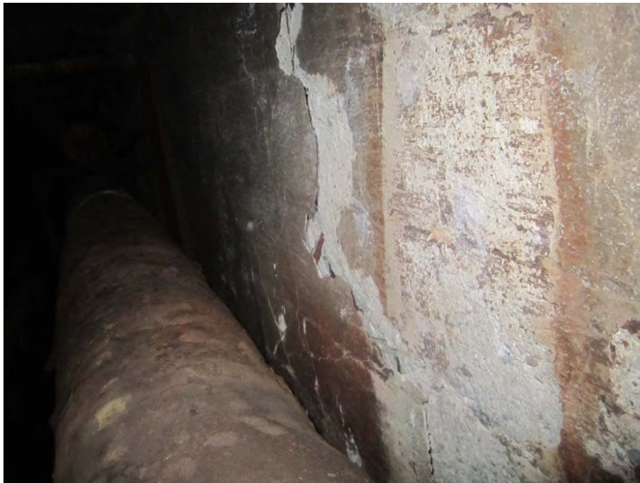
Picture #42- Shallow delaminations Section 30-31
