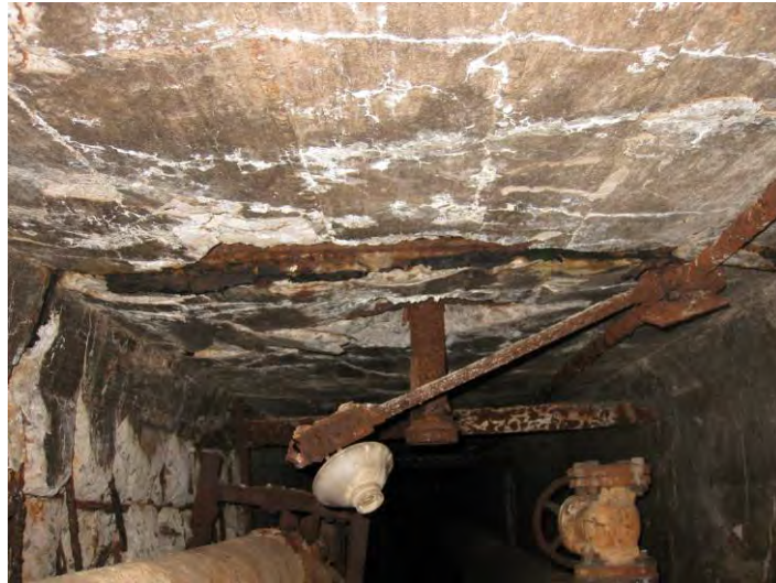
32. Tunnel's Ceiling Delamination (Concrete Ready to spall off)
