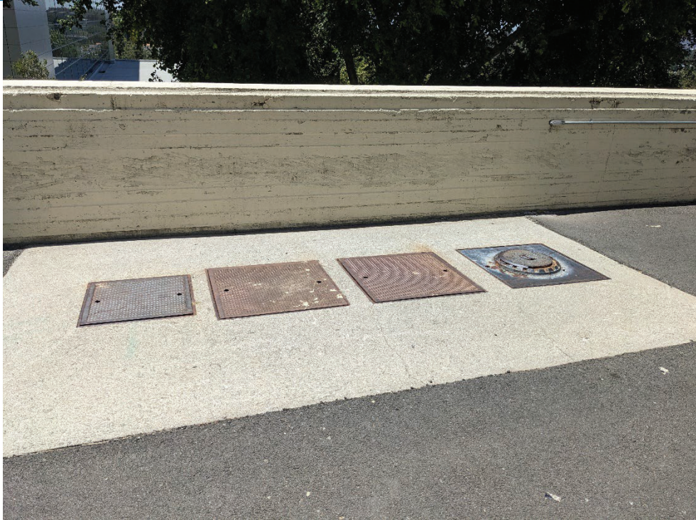
PHOTO 29: View of 4-stage cooling tower clarifier.
