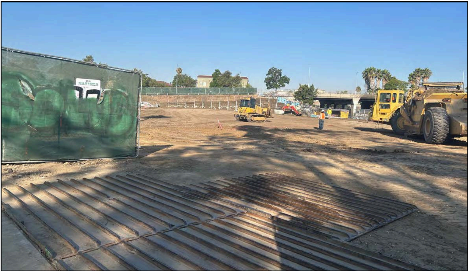
Figure 22: Construction of Project Site - Corner of N. Mission Rd. and Griffin Ave.
