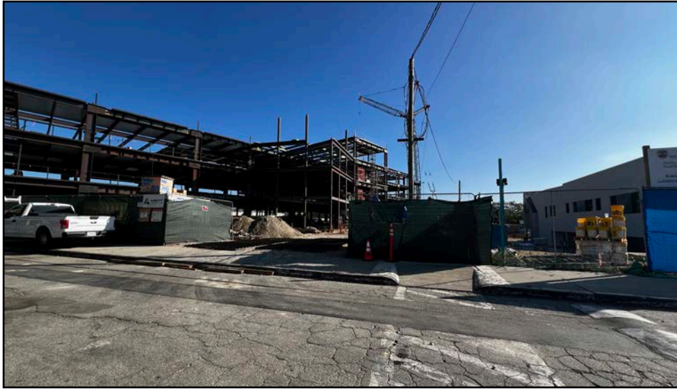
Photo 2A: Active construction area near the intersection of N Mission Rd and Zonal Ave.
